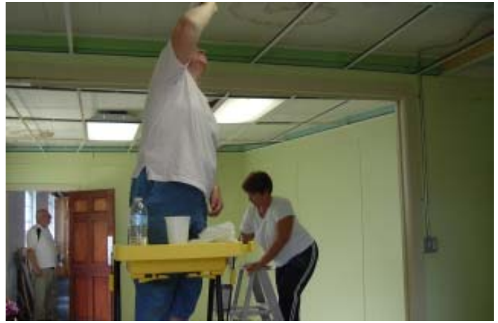
Charlene and Cathy painting the metal framework in preparation for new ceiling tiles.
